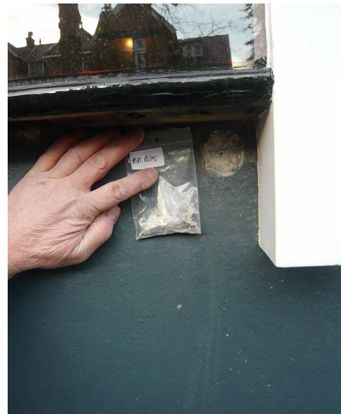
FIG. 3.19 Plaster sample from the wall below the studio window on Prins Hendriklaan
