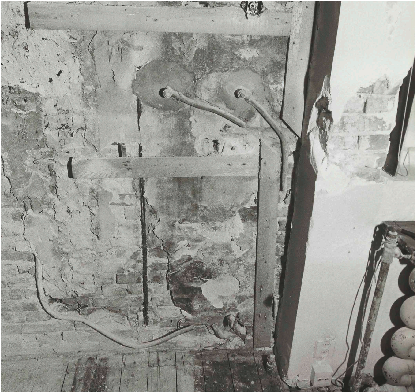
FIG. 3.1 The dismantling of wall, floors and ceiling yielded a lot of information about pipes, connection points and the attachment of furniture
