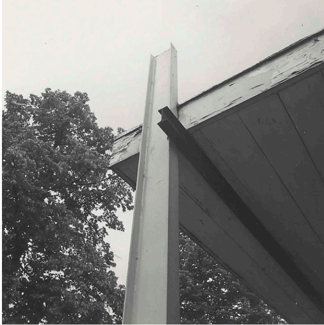
FIG. 1.4 Unconventional constructions made the house vulnerable
