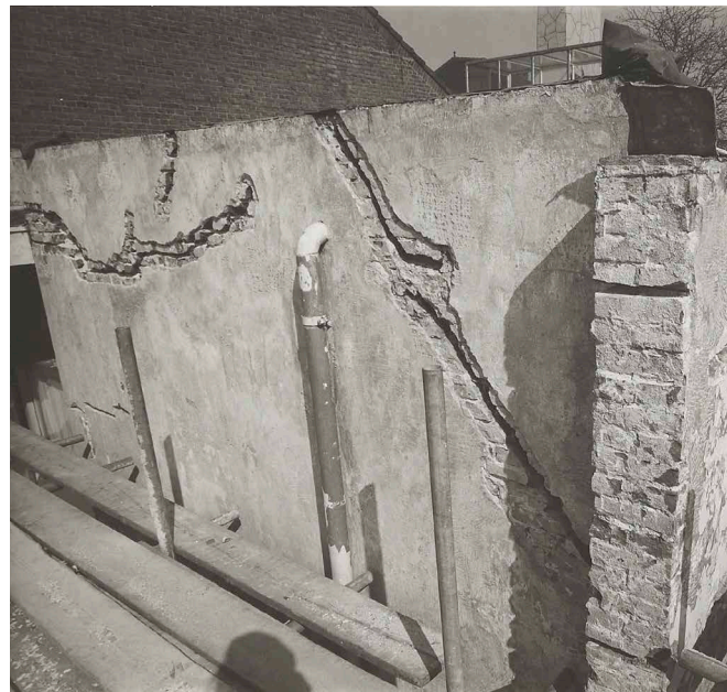
FIG. 1.9 The brickwork displayed deep cracks
