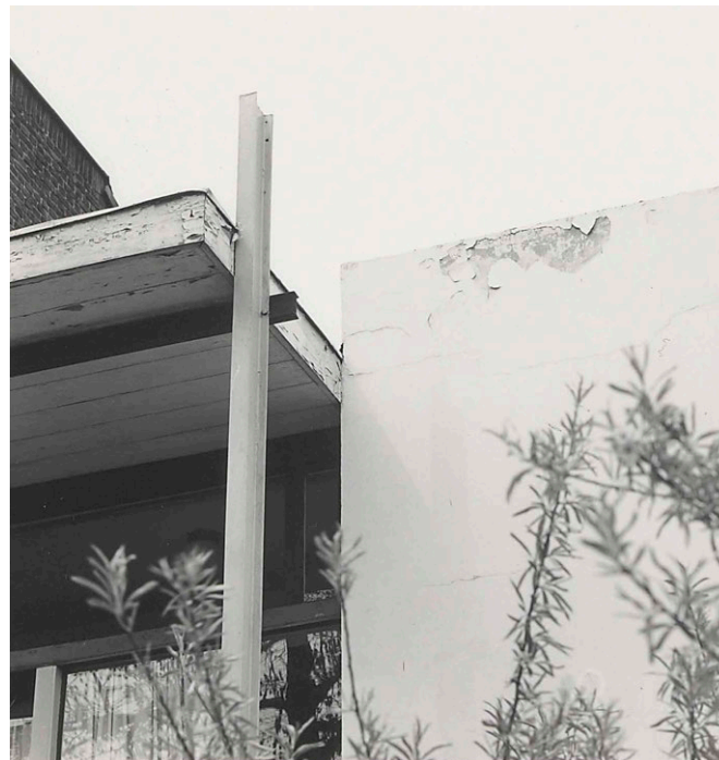
FIG. 1.3 Plasterwork and wood exhibited serious blemishes
